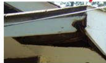
ROTTING SOFFIT & FASCIA
