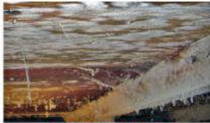
MOLD & MILDEW IN THE ATTIC
